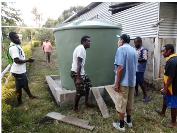
New water tank
